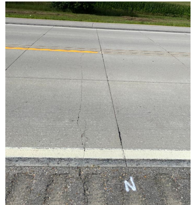
Crack near undeformed joint (aligning with major reflective crack)
