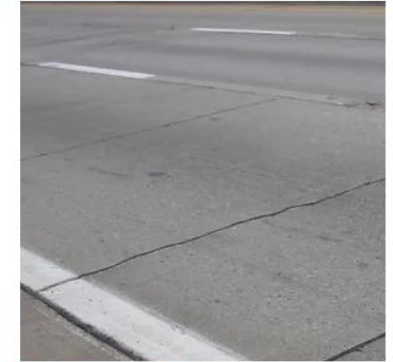
Low-Severity Transverse Cracks
