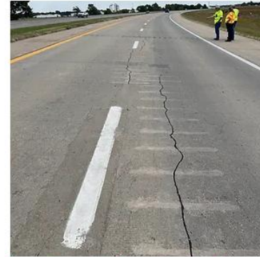
Low-Severity Longitudinal Cracks or Joints
