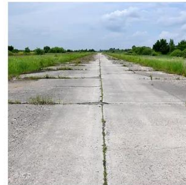
Joint Sealant Failure
