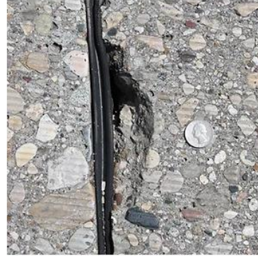
Spalled Joints and Cracks
