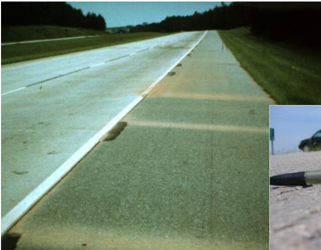
Loss of Fines (Pumping)
