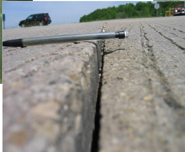
Transverse Joint Faulting
