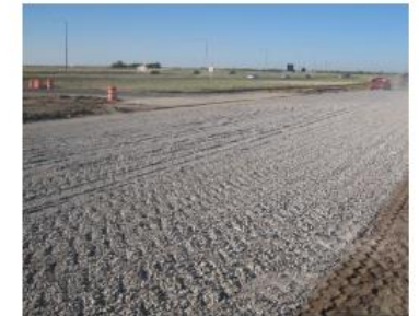
Figure 1. Rubblized surface prior to placement of the 2-inch CDOT Class 6 aggregate base.
