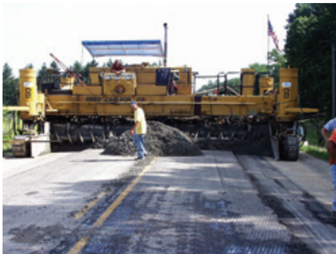
This project in Delaware County, Iowa, is called a “reverse Oreo cookie” because asphalt is sandwiched between two layers of concrete.
