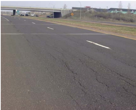
Fatigue cracking on TH 52 asphalt pavement.
