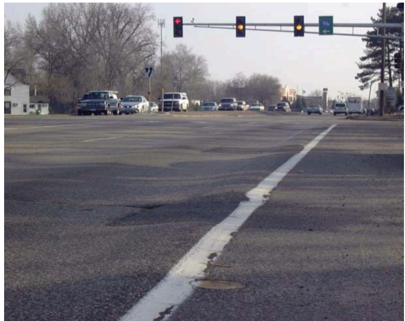
U.S. 61 Asphalt Overlays— 3 overlays in 28 years and looking rough.
